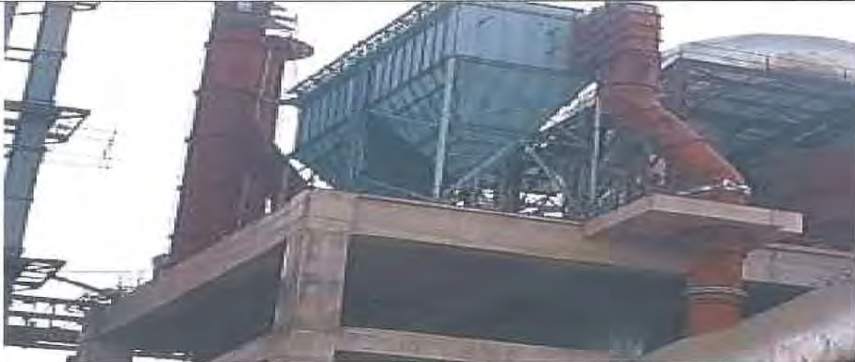
Bag Filter installed
